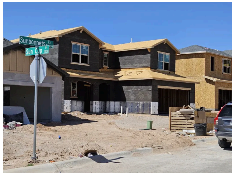
Homes under construction in the Campo Del Sol housing development in far Northeast El Paso. (Daniel Perez / El Paso Matters)
