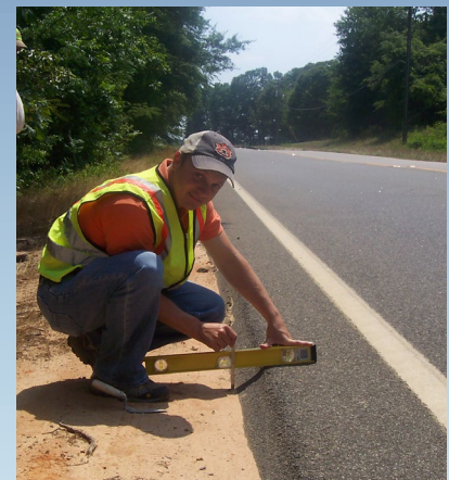
Example of SafetyEdge SM after backfill material settles or erodes. Source: FHWA
