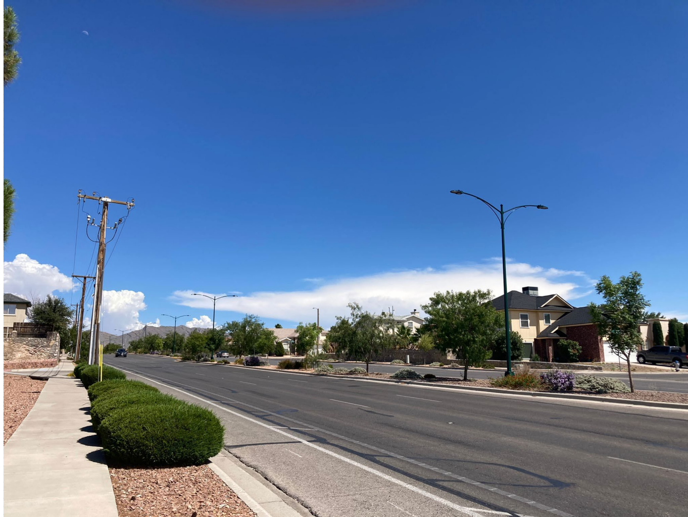
Current condition on previous improved section at Resler Dr. and Helen of Troy Dr.
