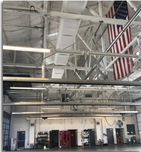
Fire Station 5 Vehicle Exhaust
